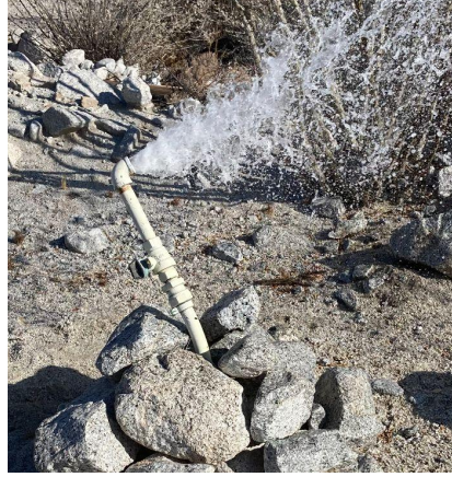
Replace Brittle Blow-offs
