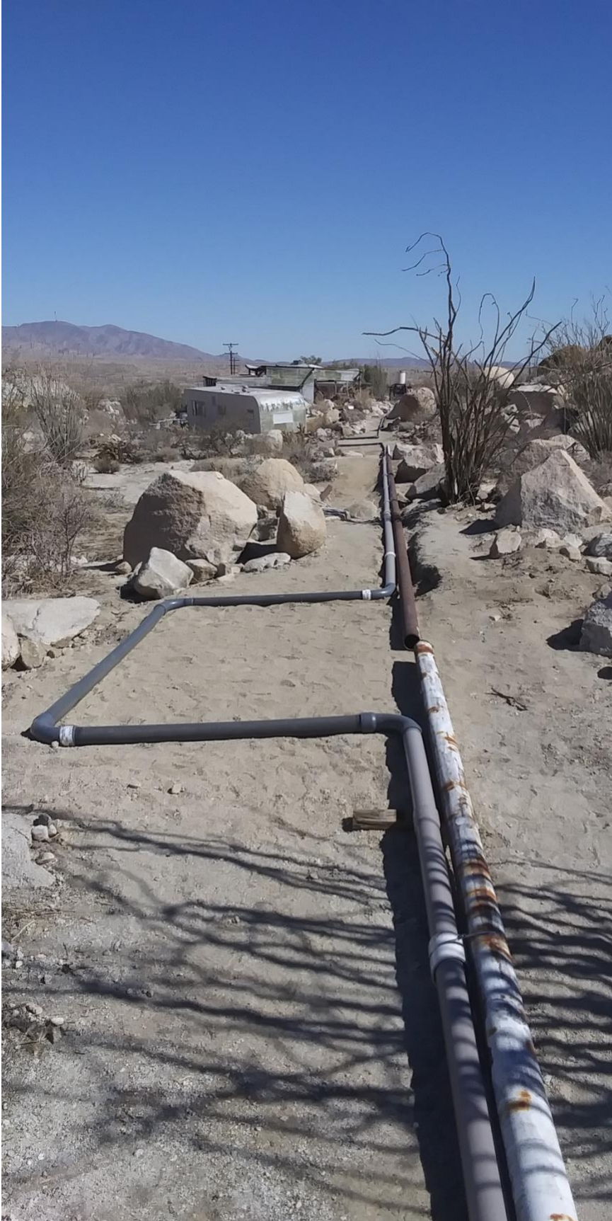
Close-up of expansion loop
